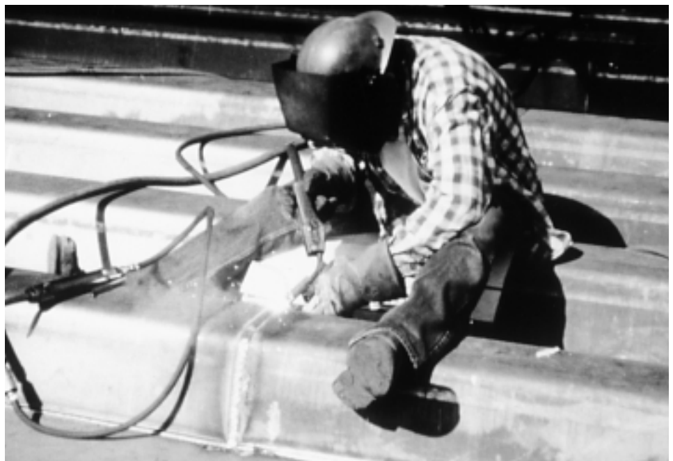
Figure 3. Semi-automatic welding was needed to provide continuity at ends of ribs fabricated in 20 ft (6 m) long straight segments tangent to radius.
