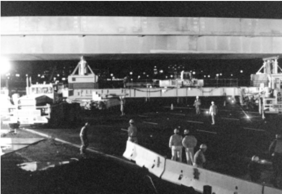
Figure 4. Special heavy-lift hydraulic platforms (SHLHP) pull a 450-ton (408 m ton) all-steel orthotropic section across freeway lanes.
