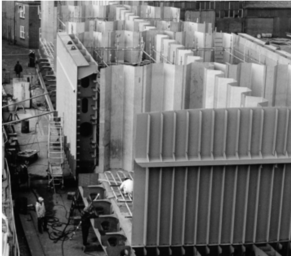
Figure 2. Actual view of the layout of the tanks.
