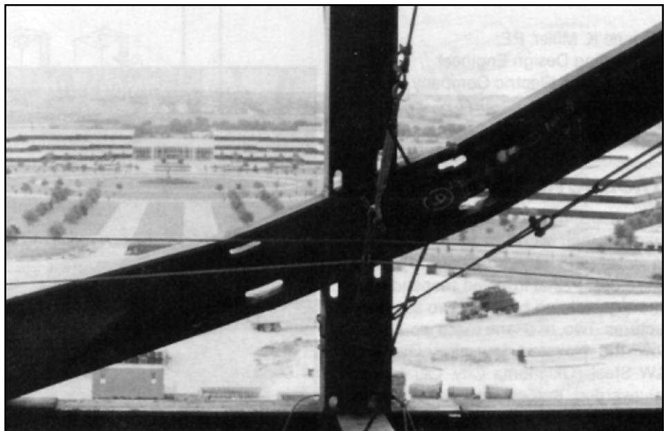
Figure 3. Access holes can become large. The location of field splices allows for shop fabrication of the most difficult assemblies. Note the EDS campus in the background.
