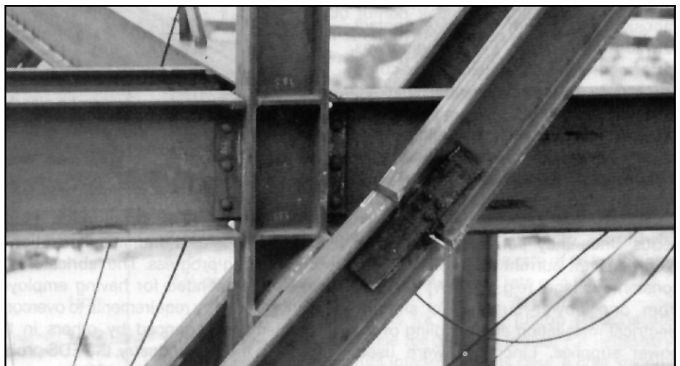
Figure 2. The non-planar orientation of the catenary would have made bolted connections difficult or impossible to achieve.
