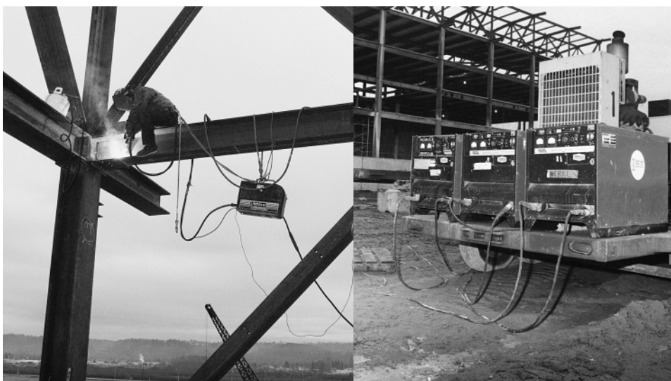
Figure 2. The arc voltage is always lower than the machine voltage due to the resistance of the welding cables.
