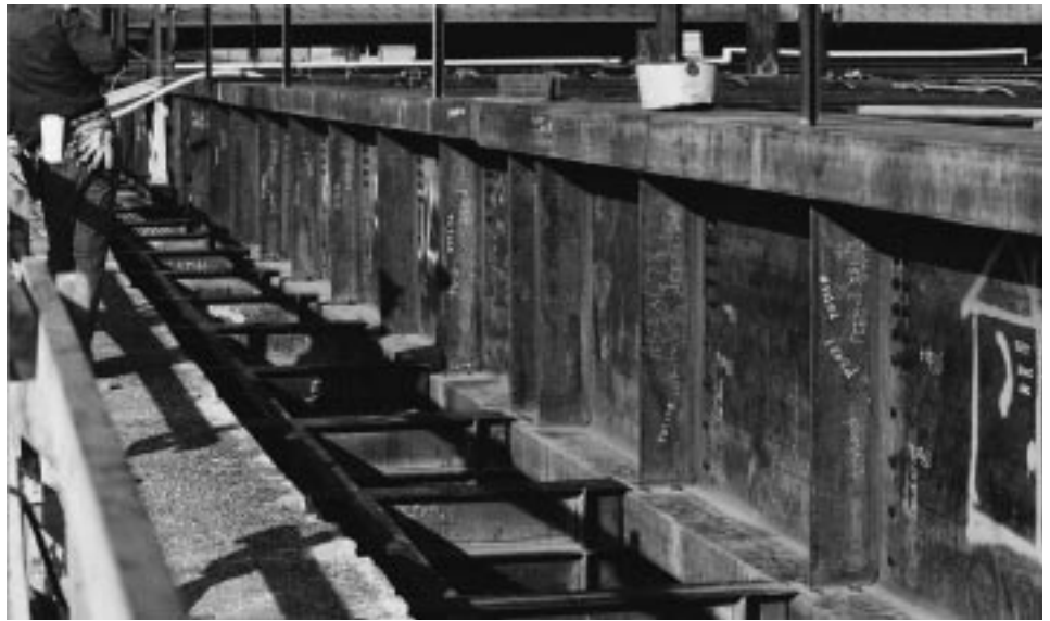
The 7 in (180 mm) flanges of these transfer girders require careful consideration of the NDT acceptance criteria.
