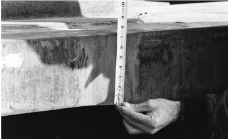
Heavy sections may require especially rigorous alternate acceptance criteria.
