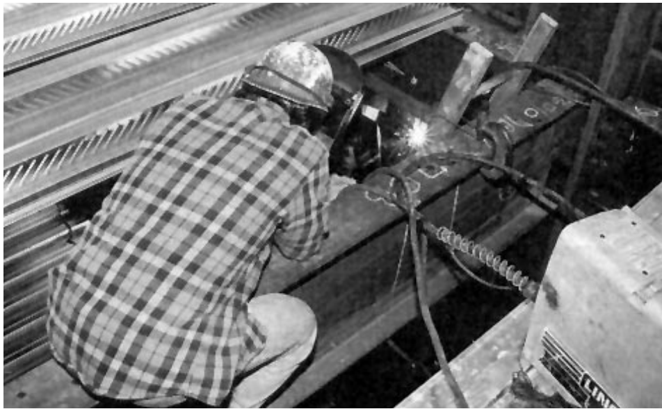
Effective visual inspection requires that the Inspector be present when welding is being performed.
