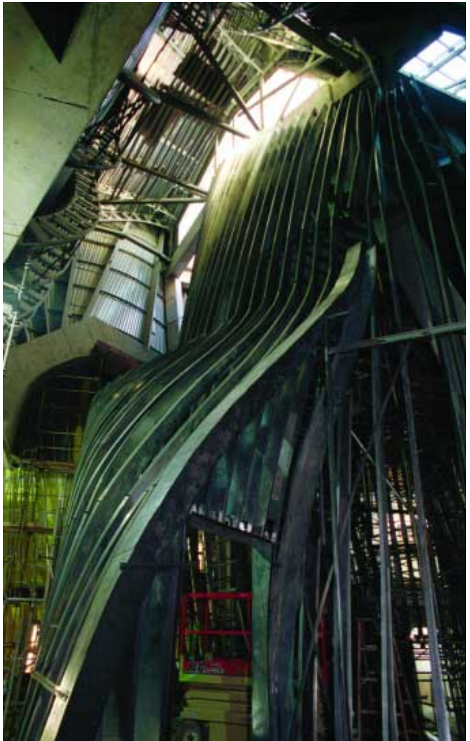
This soaring structural steel framework is now hidden by the outer skin and inner walls of the building.
