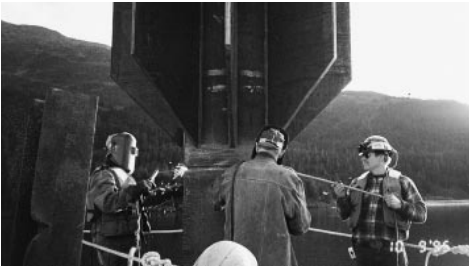
Figure 2. Field splicing the anchor pile. The API 5LX-60 steel required pre-heating and interpass temperature control throughout the welding operation.
