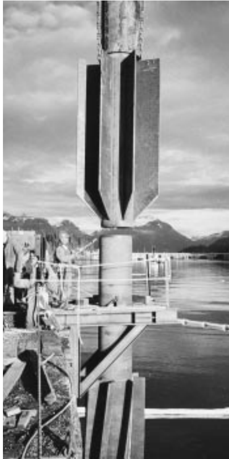
Figure 1. The two sections of the anchor pile were brought together for the welded field splice.
