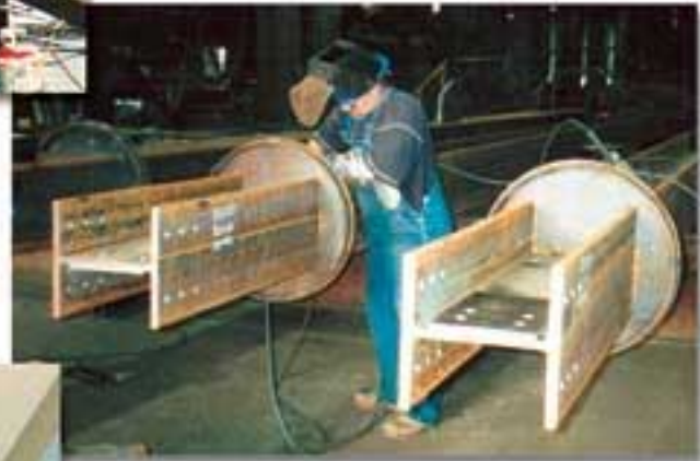
Figure 5. Shop photo showing seal welds being placed around the lid assemblies used for waterproofing.
