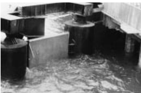
Figure 3. This close-up of the wave barrier under construction shows the concrete panels. Note the perpendicular extension of the heavy steel cap beams to the barrier piles.
