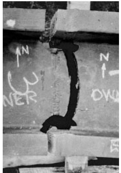
Figure 4. Wide flange section weld access hole crack.
