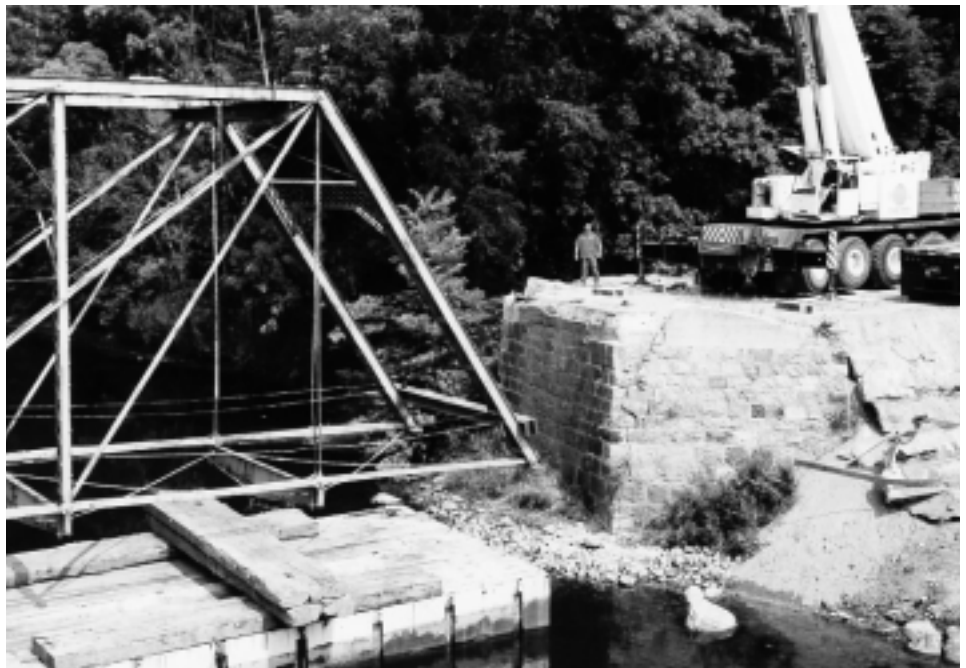
Figure 3. Lifting the Charlotte Highway bridge from its original abutment. This end was lowered onto a barge prior to hauling the bridge across the river and up the other bank.
