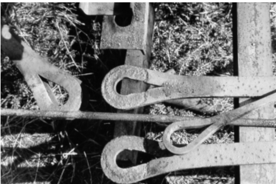
Figure 5. Forge-welded loop eye-bars like these are obsolete.
