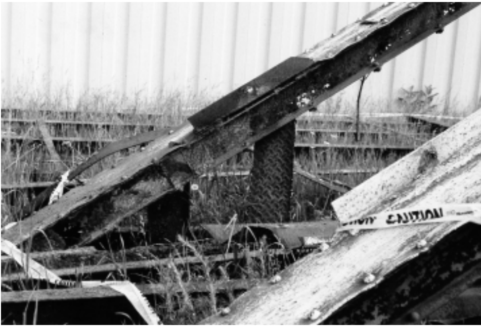
Figure 4. Severely corroded sections of the Twenty Mile Road bridge were replaced by welding new steel to sound original material.
