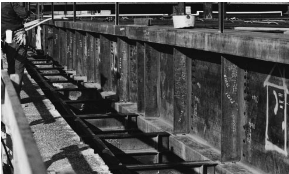
Figure 2. The 7” flanges of these transfer girders require careful consideration of the NDT acceptance criteria.
