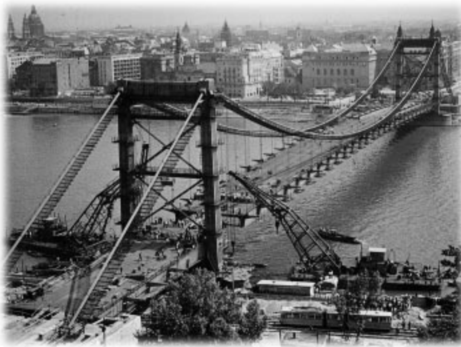
Figure 4. This photo shows the last 100 tonne deck unit of the Erzsébet cable bridge being set into place in 1964.
