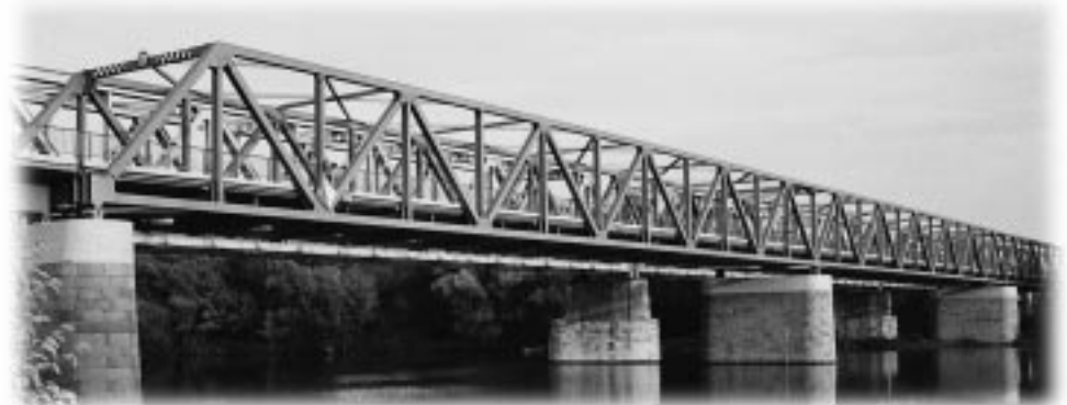
Figure 3. The welded lattice girder composite bridge over the Tisza at Tiszafüred is composed of spans measuring 30.0 + 3x70.0 + 30 m.
